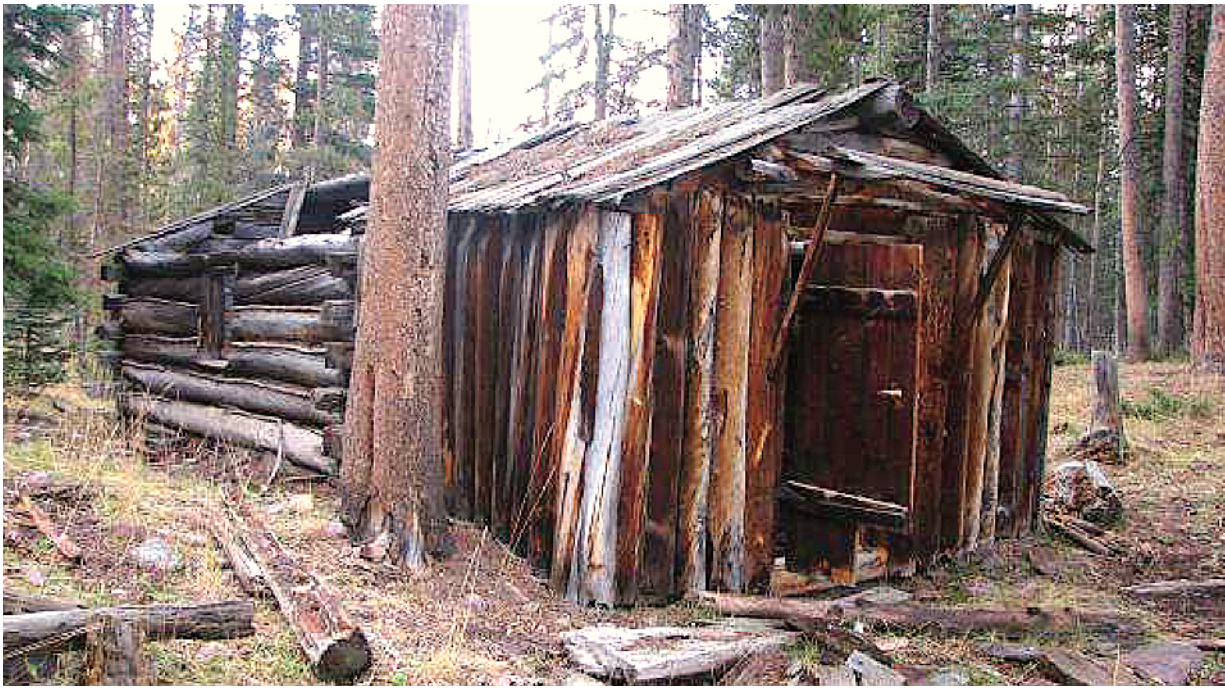
Figure 12.3 —Cabin used by a railroad tie cutter in the Uinta-Wasatch-Cache National Forest, Utah. Such historic structures are highly susceptible to damage from wildfire (photo: C. Merritt, Uinta-Wasatch-Cache National Forest).
