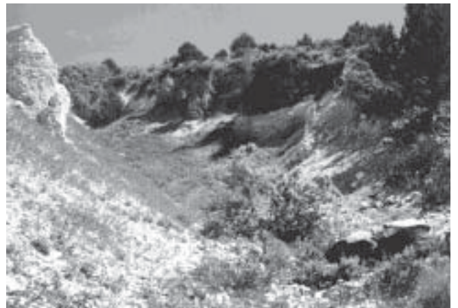
Figure 5 —Blueleaf aster stabilizing a severely eroded cut.
