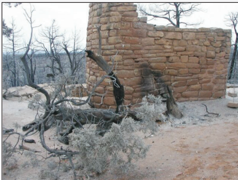
Figure 9S-5c —Damage to a sandstone wall caused by direct flame contact during the 2002 Long Mesa Fire, Mesa Verde National Park, Colorado.
