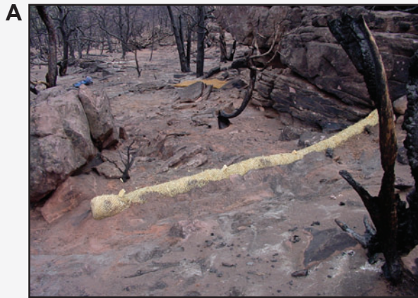
Figure 9-S4.a —Burned Area Emergency Rehabilitation work to protect a rock shelter following the 2002 Mustang Fire, Ashley National Forest, Utah. Straw wattle (foreground) was used as a runoff barrier to protect the rock shelter from water coming in from the side, which could result in erosion damage. An erosion blanket (brown patch in mid-ground) was used to protect the floor of the rock shelter from water flowing off of the overhanging ledge (Johnson 2004a,b) (photo August 2002, by Clayton Johnson, USFS Ashley National Forest).
