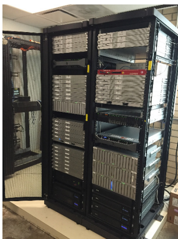
Figure 2: The FireBuster forecast model runs on a 40-core Dell PowerEdge R820 server. Mass storage systems are used for archived data. Another server (not shown) converts model output to web-displayable graphics.
