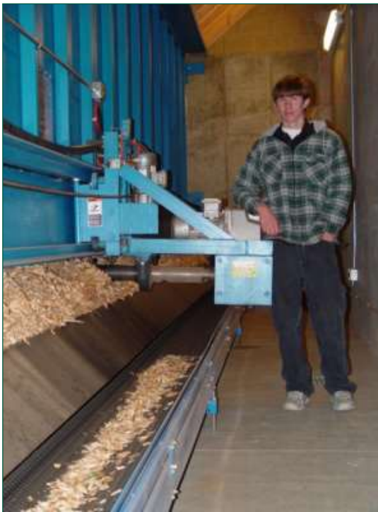
Wood chips ride a conveyor to Darby School's new biomass boiler. This alternative reduces school heating costs and effects associated with open burning of excess forest fuels. (Photo courtesy of USDA Forest Service.)
